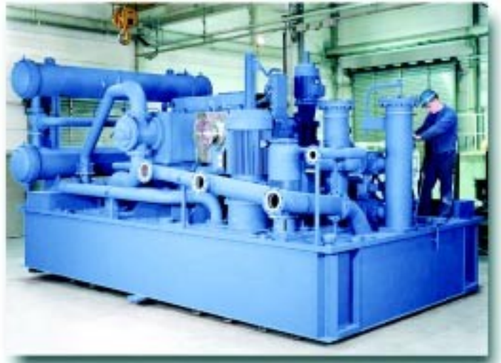
Main and standby NSS pumps on lubrication service
