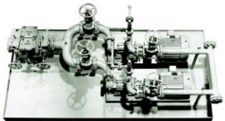
Main and standby 3D-218 fuel pumps on common skid with inlet strainer, discharge relief valves and block valves.
