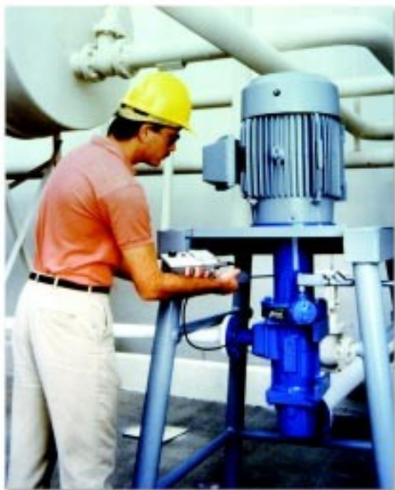
Vertical, magnetic drive 3D-250 pump on chemical service
