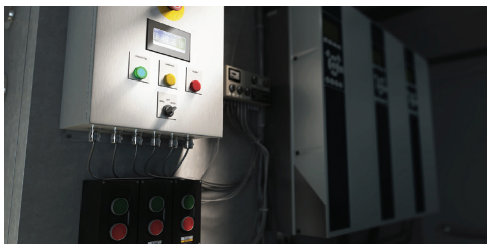
RIGHT: The intelligent controller has realised savings of more than 455,000 kWh for the two seawater pumps on Kyoto Express
