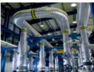
UNLOADING TRANSFER & FUEL FORWARDING
