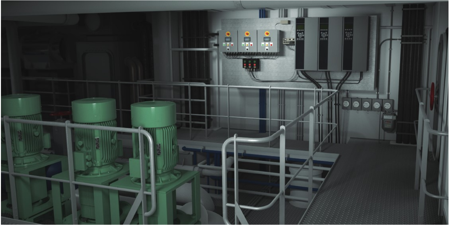
This typical engine room demonstrates the placement of three cm-1000 intelligent controllers in a 3 x 50% pumping configuration. Individual pump controllers ensure optimum energy savings and reliability.
