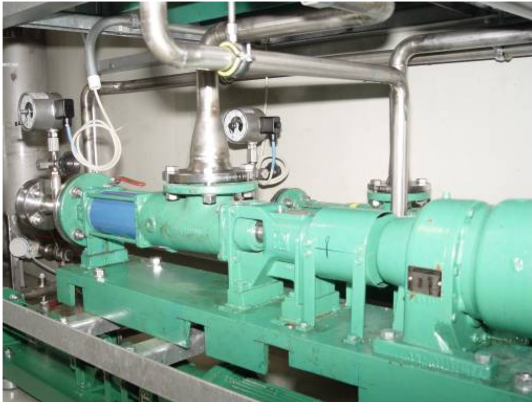
ALLWEILER progressing cavity pump for moving glycerin phase, discharge pressure 2 bar, capacity 6 m 3 /h.
