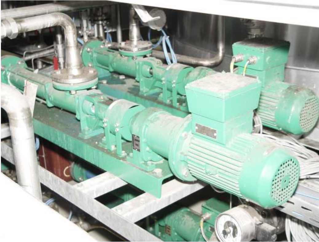
ALLWEILER progressing cavity pump for moving glycerin phase, discharge pressure 1 bar, capacity 1.3 m 3 /h.
