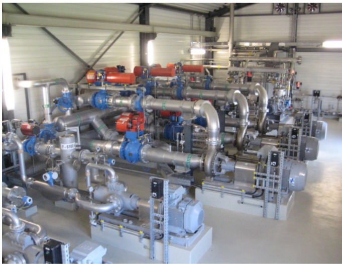
Allweiler pumps in the Matzen extraction station's pump house. In front a screw pump for pumping crude oil; behind that three centrifugal pumps for pumping formation water.
