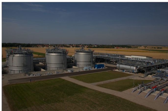
The tanks for the A and P qualities and a reserve tank each hold 1000 m 3 . The two water tanks hold a total of 2000 m 3 . All of the tanks are fed by Allweiler pumps.
