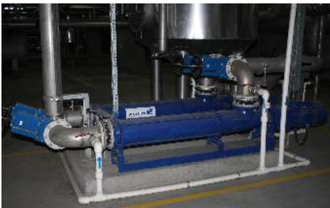
Application: Sludge transfer Pump series: ALL-OPTIFLOW® AEB1F Pump size: 5503 Flow: 100 m 3 /h / 440 gpm Pressure: 3.5 bar / 50.8 psi
