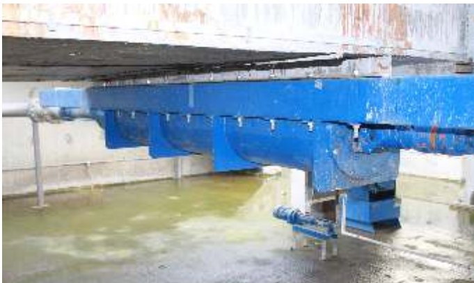
Application: The large pump moves 20-25% sludge from silos to dryers. The small pump proportions are used for polymer injection in the discharge pipe for reducing pressure losses.
