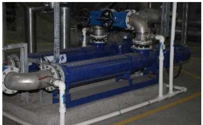
Application: Sludge transfer Pump series: ALL-OPTIFLOW® AEB1F Pump size: 5503 Flow: 100 m 3 /h / 440 gpm Pressure: 3.5 bar / 50.8 psi
