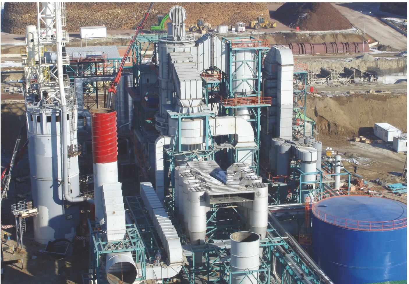
48-MW biomass-fired hot-gas generator with eight pumps for circulating heat-transfer oil and one for cooling water
