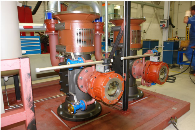
Redundant twin three-screw pumps of the SNS series in an oil-supply system (“OWGX” construction type) for an extruder drive. The pumps move synthetic or mineral oil VG320 at a pressure of 8 bar.
