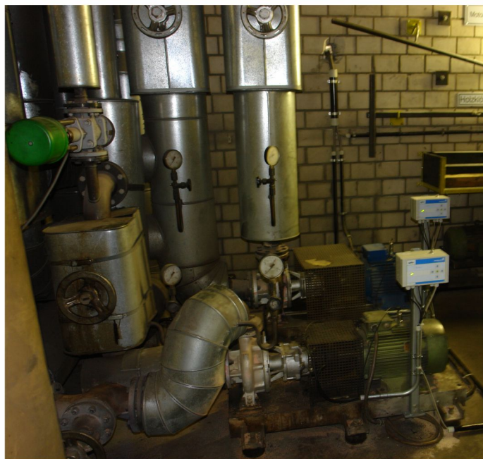
Heat-transfer units with ALLMIND installation
