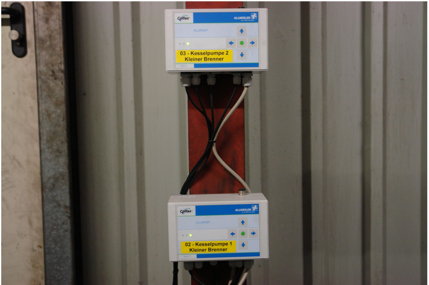
Traffic light on expansion module communicates status quickly. Details may be retrieved from the Master unit.
