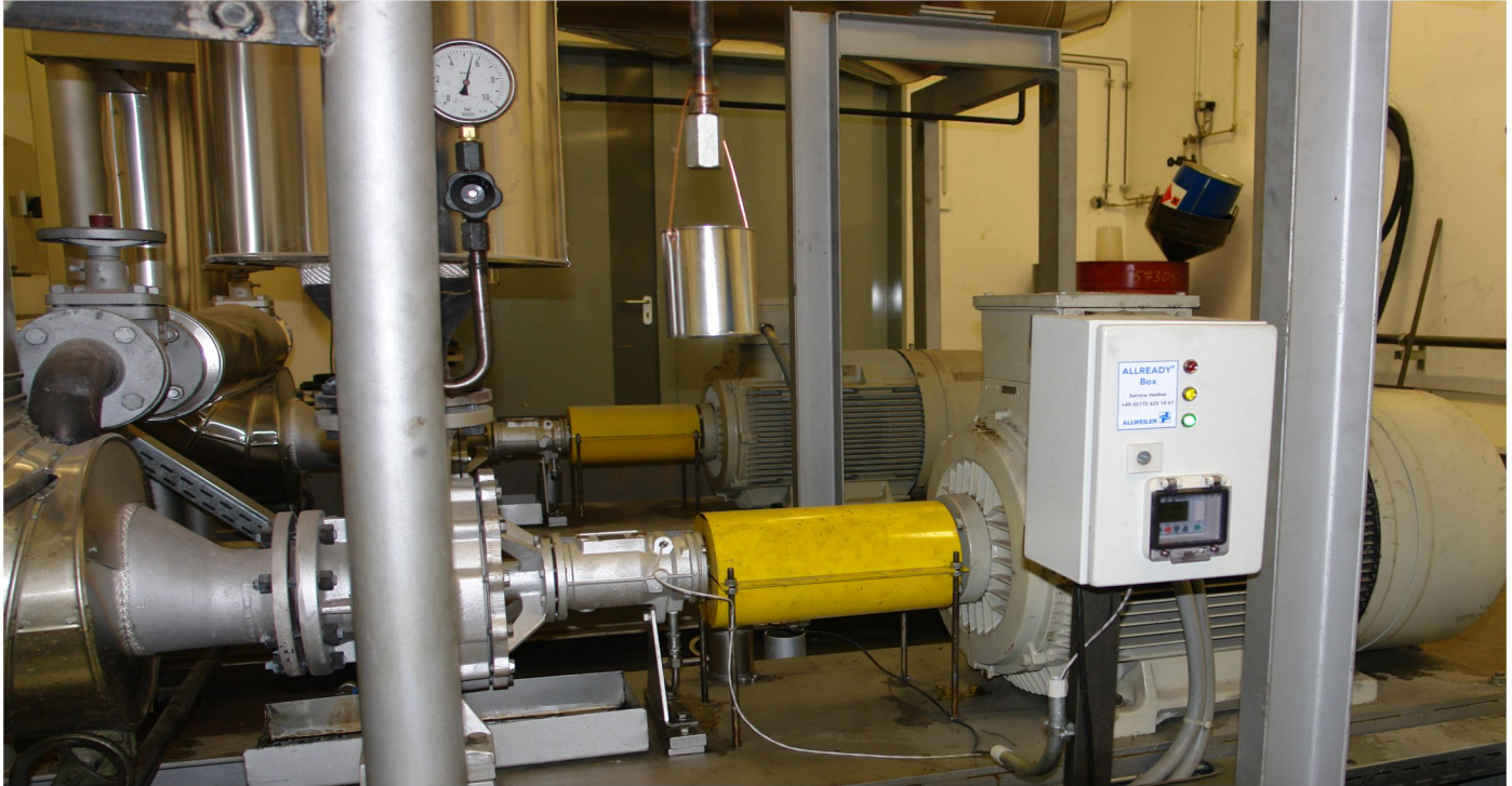
Already Box on a pump in the primary loop. The "green" lamp indicates that temperature and leaks are in the acceptable range.
