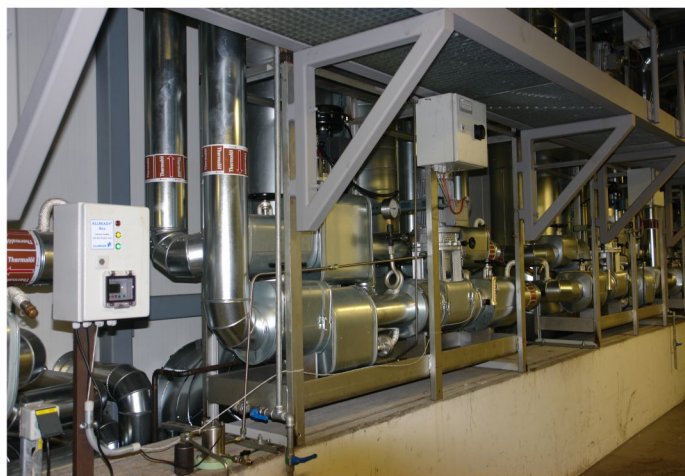
Allweiler heat transfer pump with Allready Box in the secondary loop. These units also have a green light.
