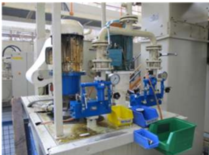
EMTEC pumps with valve-based control before the conversion.
