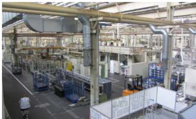
Three pumps in this production line were converted to frequency control.
