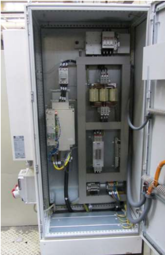
Switch cabinet with frequency converter, throttle, filter, and control logic.
